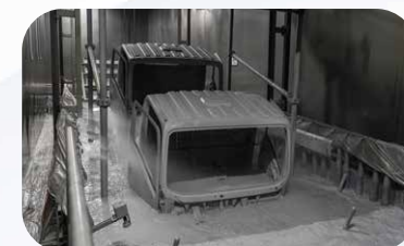
4. ED coating line
